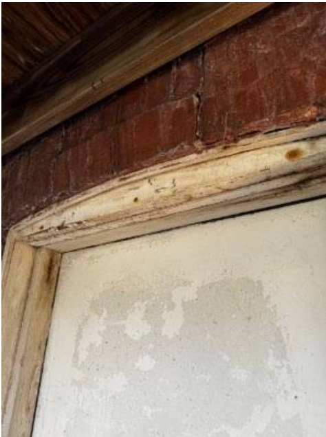
Photo 7-1 above back door basement
