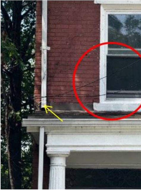
Photo 6-1 Missing extension on downspout
