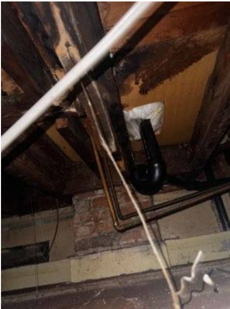
Photo 16-1 ceiling above kitchen
