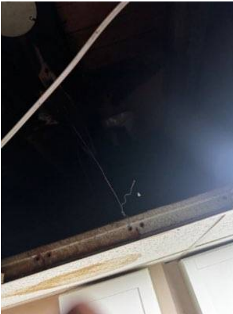
Photo 16-2 ceiling above kitchen
