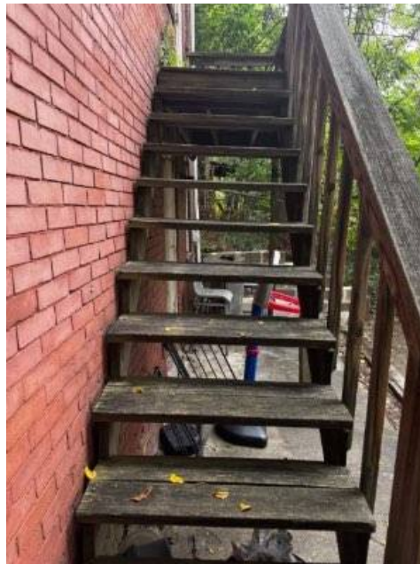
Photo 3-2 steps need powerwash and resealed
