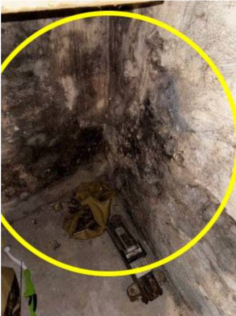
Photo 8-1 front wall right corner efflorescence
