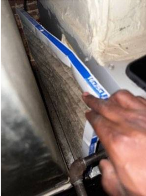
Photo 19-1 dirty filter need replace
