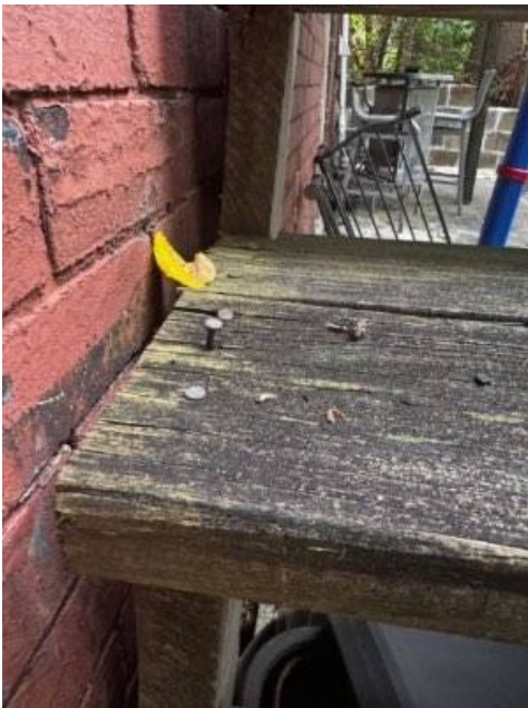
Photo 3-1 exposed nails backyard stairs
