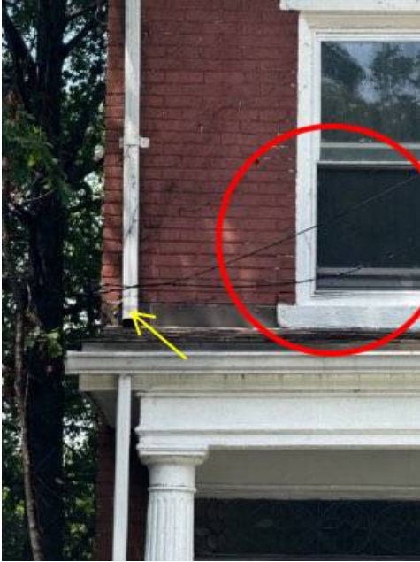
Photo 12-1 Missing extension on downspout
