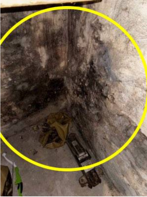
Photo 9-1 front wall right corner efflorescence
